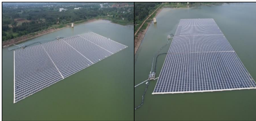
Fig. 6 : Floating photovoltaic plant on surface of Meghadrigedda reservoir
