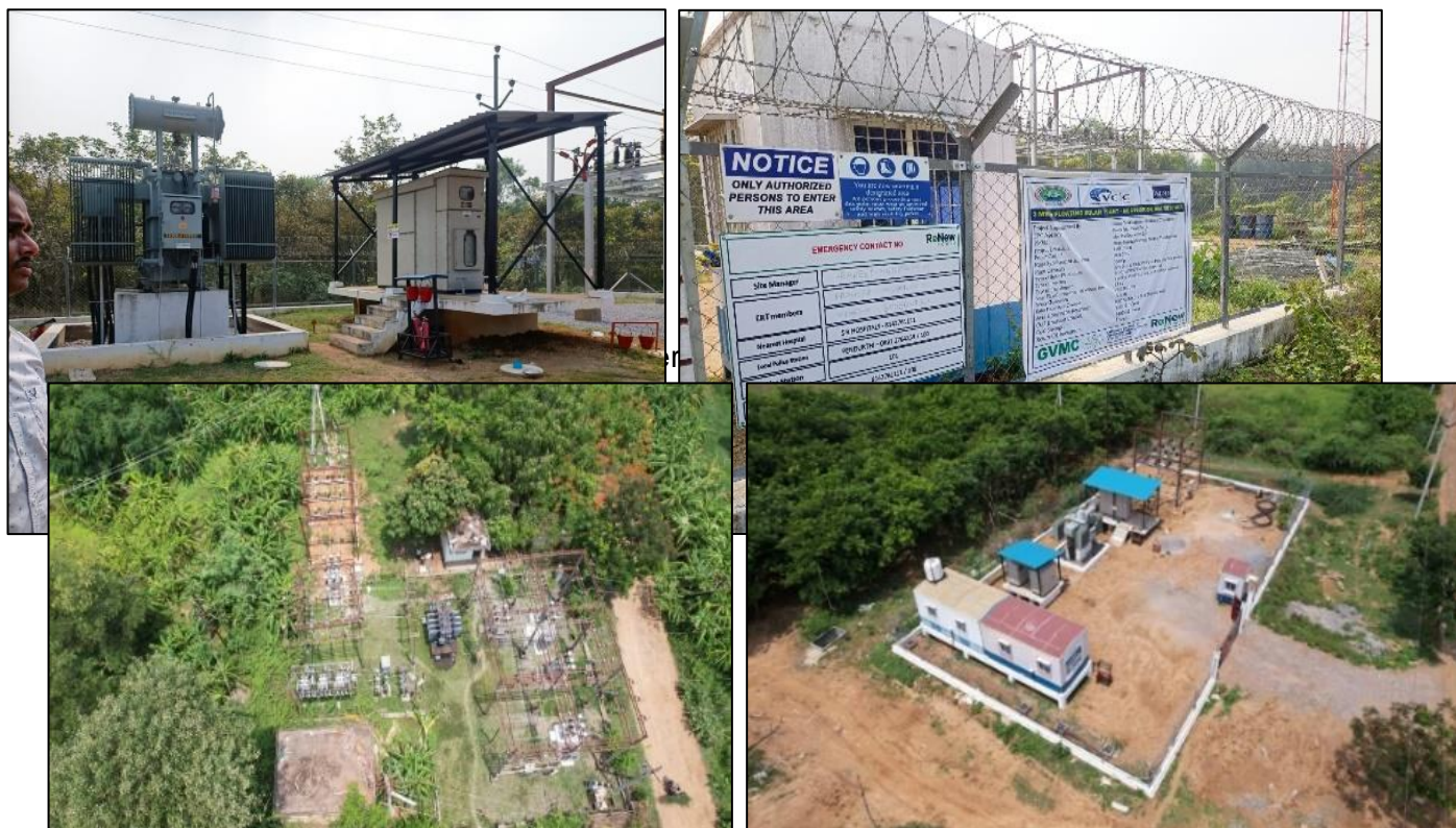
Fig.9: Aerial view of 3MW transformer installed
